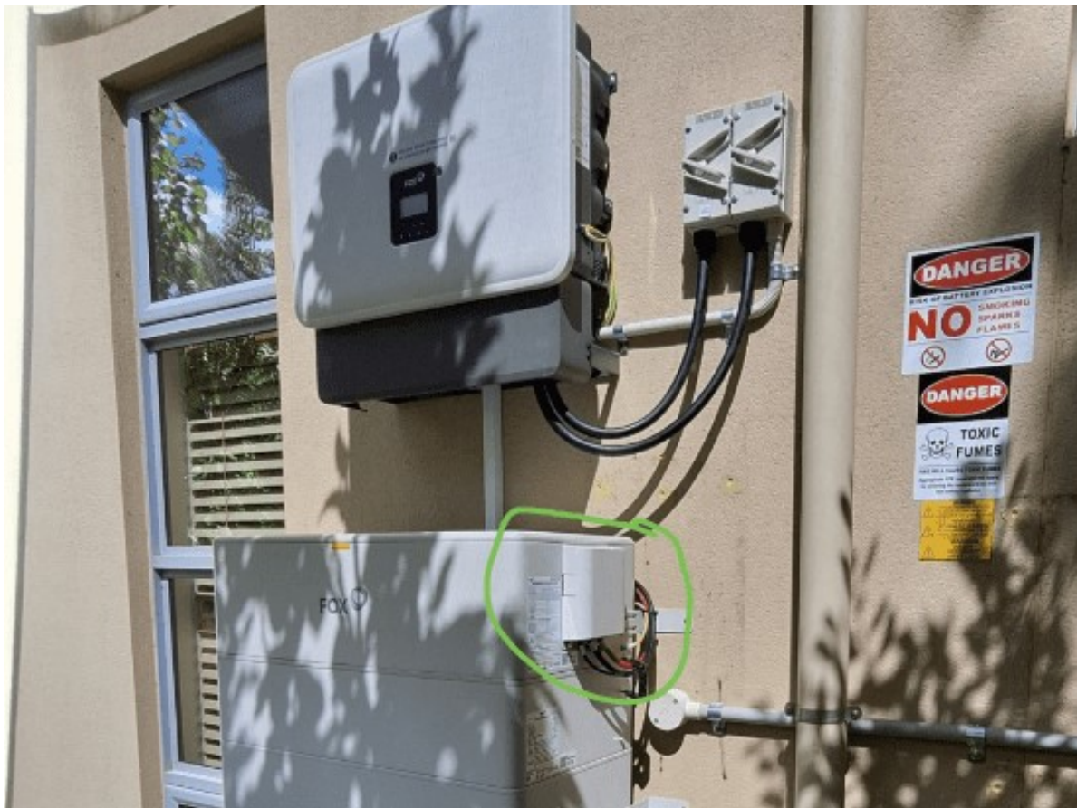
Inverter looks good: shame about the exposed DC at the battery.
