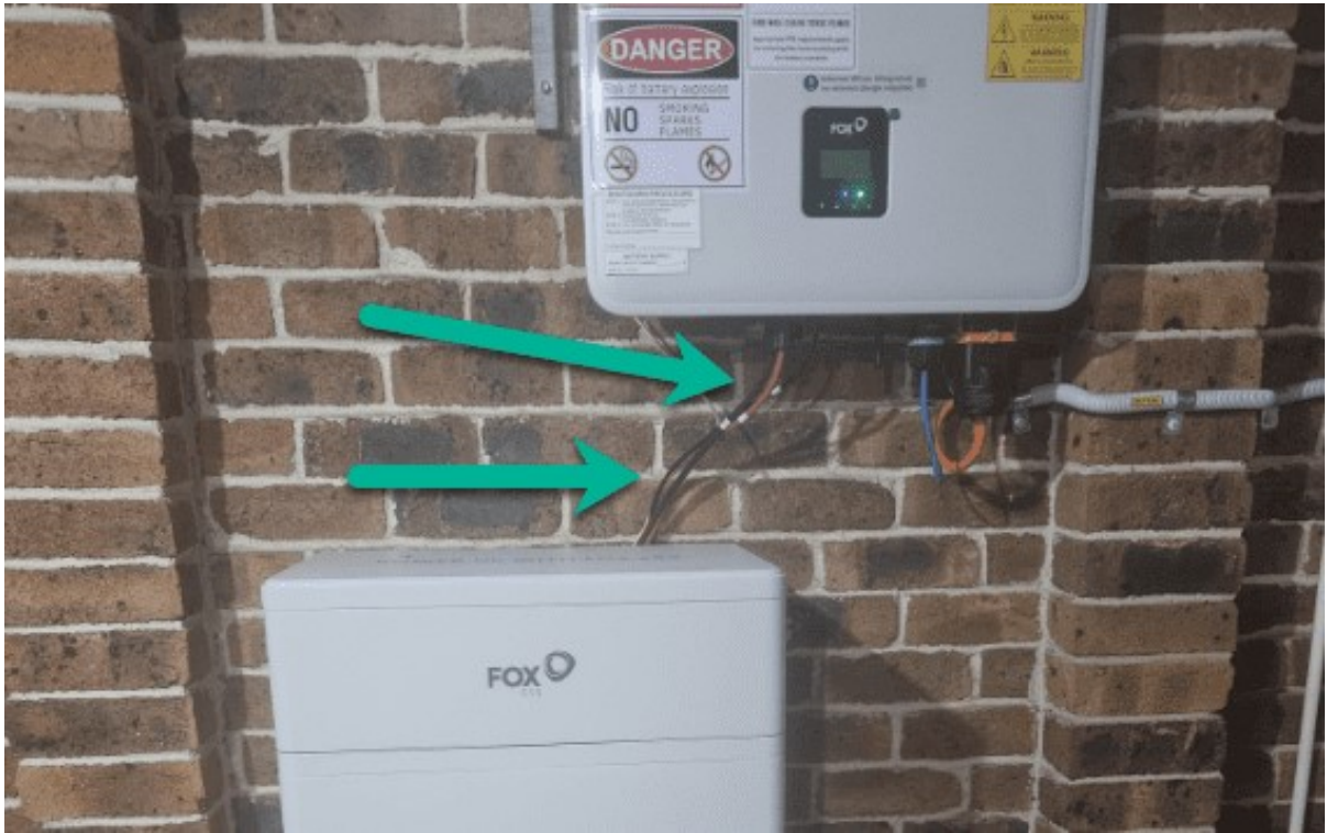
Unprotected battery cables from the battery to the inverter. Not even close to compliant.
