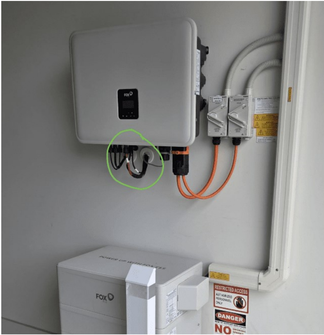
Nice and neat. Not compliant.
